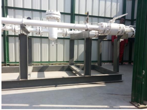
Figure 2-3: Qena current Pressure Reduction Station
