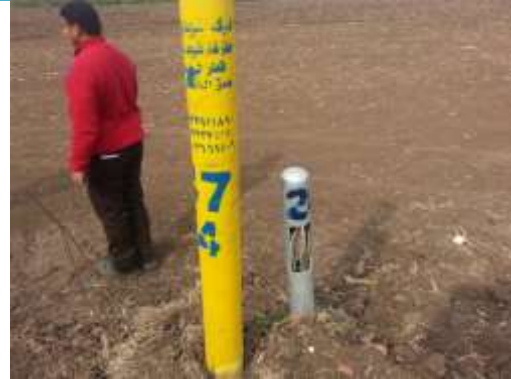
Figure 1-5: Gasco intake line
