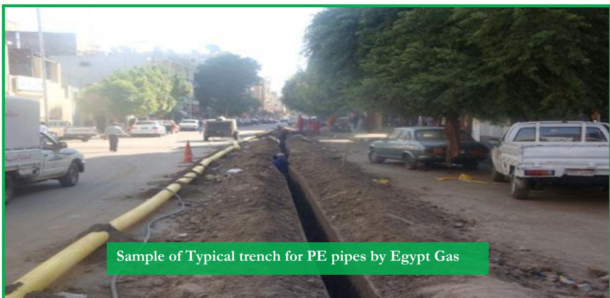
Figure 2-18: Pictures showing sample of Typical trench for PE pipes by Egypt Gas
